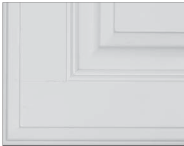
Example of front joint separation
