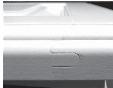
Example of end joint separation
