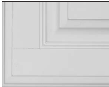
Example of front joint separation
