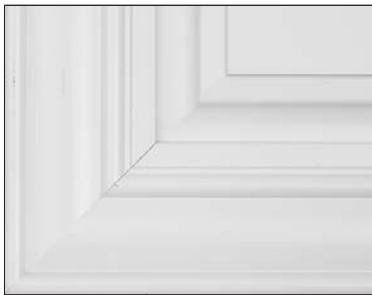
Example of front joint separation
