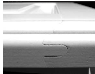
Example of end joint separation
