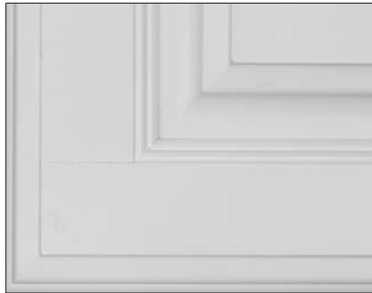
Example of door front joint separation
