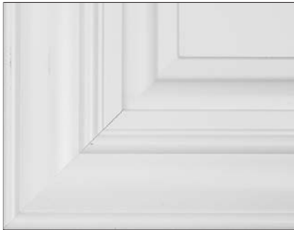
Example of door front joint separation
