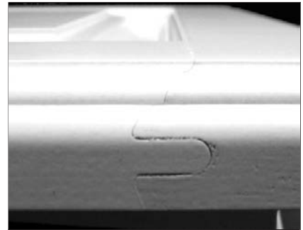
Example of door end joint separation
