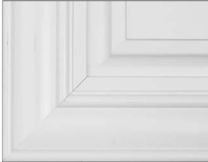
Example of door front joint separation
