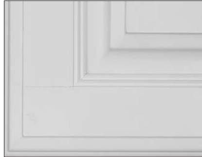
Example of door front joint separation
